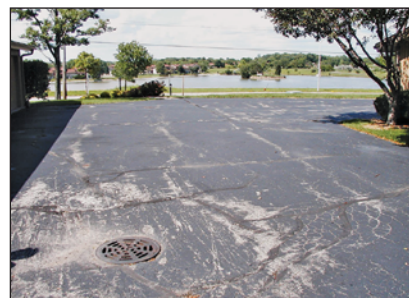
Light gray patches of asphalt show where sealcoat has been worn from the pavement. Applicators recommend reapplication of sealcoat from every 1 to 5 years. 1
